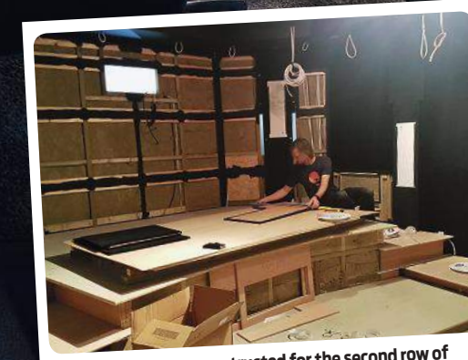
A raised floor was constructed for the second row of cinema seating. Behind, on the rear wall, space has been allocated for installing the JVC projector
